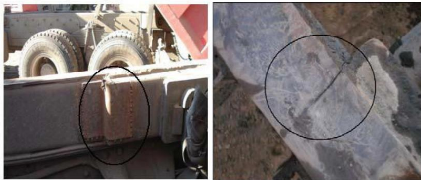
Fig.3.1.1 Fatigue crack of the sub-frame
